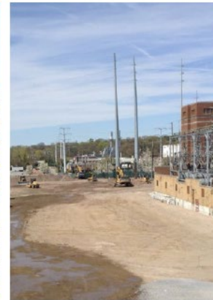
Glenwood Landing Generating Station
