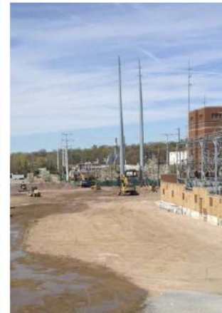
Glenwood Landing Generating Station
