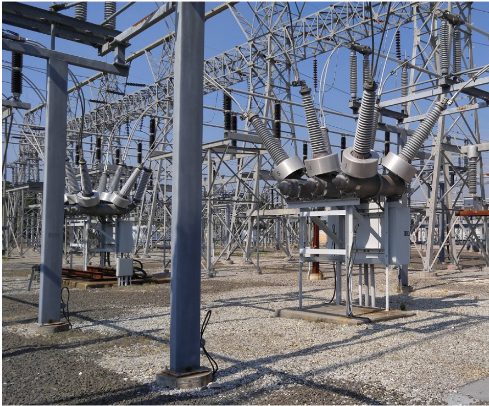
Figure 4-3: 6DL Pilgrim Replacement Gas Circuit Breakers
