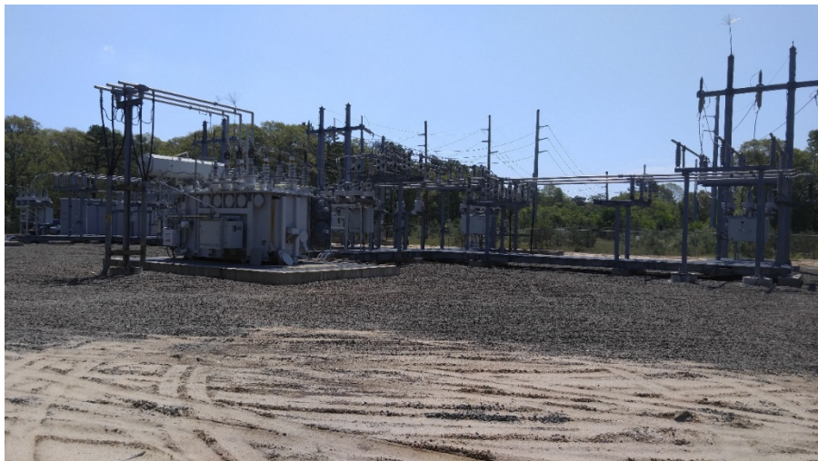
Figure 4-2: Bare Ground Spots within Substation
