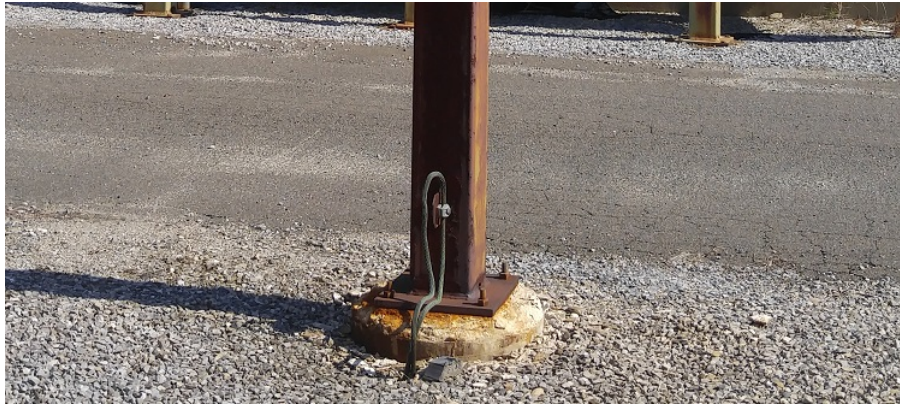
Figure 4-1: Piling Cap Deterioration
