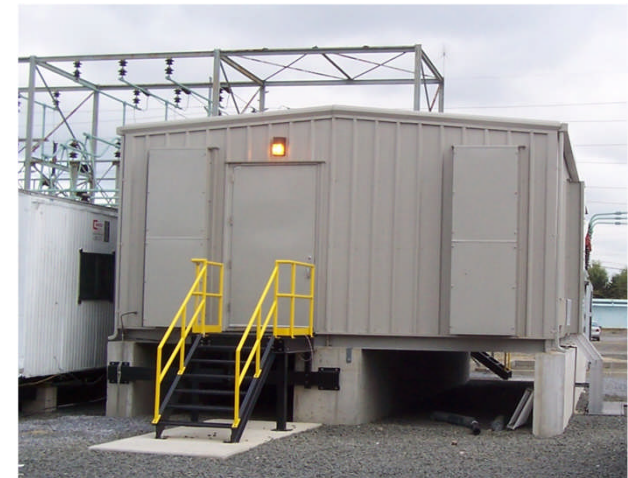
Barrett Control House - Photo courtesy of National Grid
