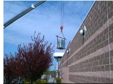
Hoisting a PV array onto the roof of Citibank Park, home of the L.I. Ducks.
