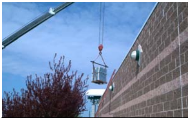
Hoisting a PV array onto the roof of Citibank Park, home of the L.I. Ducks.
